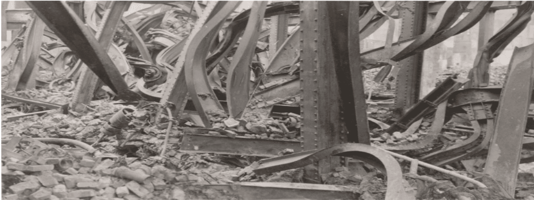
Steel after building fire
